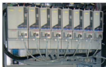
I D6 Drives & Controls
